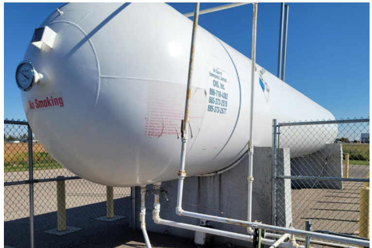
Photo taken prior to disconnection
