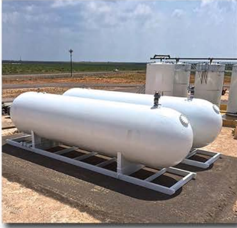
NGL Storage & Handling
